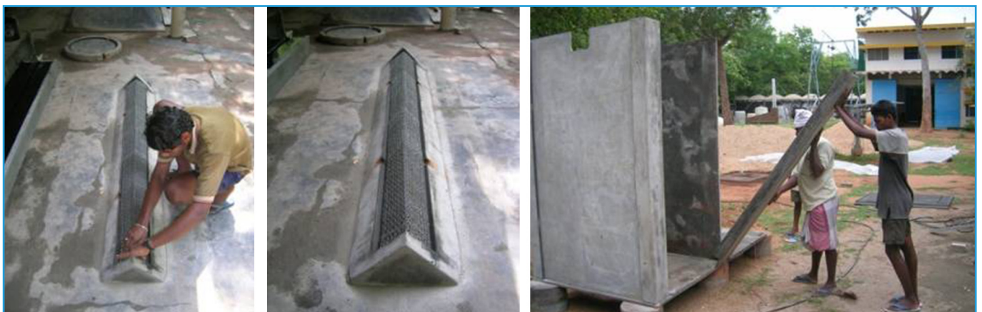
Figure 15 Casting and erection of ferro-cement for a community toilet (Sholingur, Tamil Nadu)
